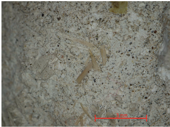
• Fig. 6. Microscope image showing the 12th century plaster consisting of lime mixed with quartz sand and straw
